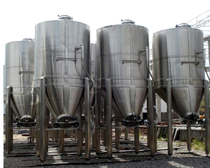
Installations in communicating vessels.
