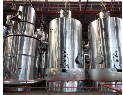
Installations in communicating vessels.
